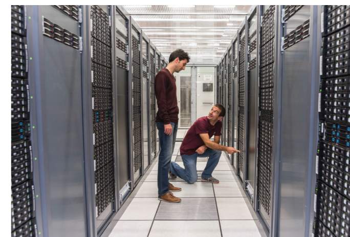
The goal of the project with Comtrade is to simplify the usage, installation, and maintenance of the EOS large-scale storage system, as well as adding support for new platforms.
